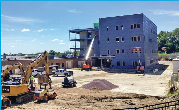
Pictured: View of progress as of 8-6-2024. Exterior framing and installation of insulation panels was ongoing. Ductwork and plumbing work was occurring and the Northeast parking lot was still being worked on.
