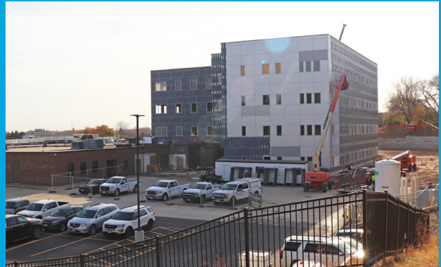
Pictured: Progress as of 10-29-2024. Metal panels are being installed on the exterior of the building, with drywall projects occurring throughout. The West parking lot is now in progress!
